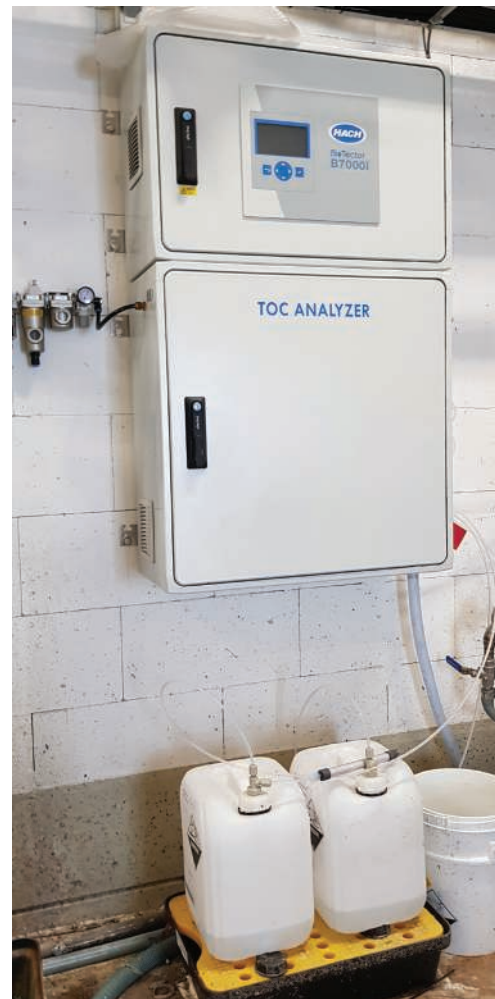
Installation of the TOC Analyzer Hach BioTector B7000i at Steinbeis.
